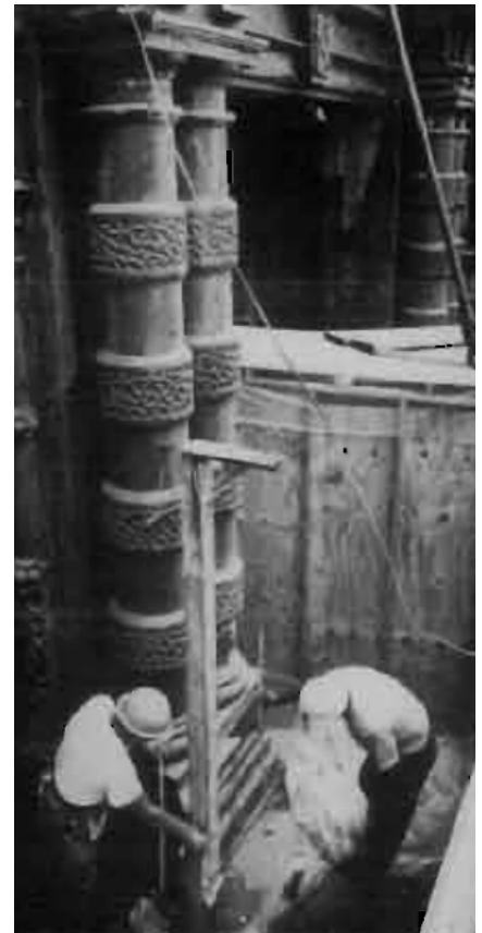
The cast iron columns of this theater are being repaired during rehabilitation.
